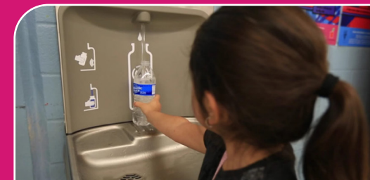
Sugar sweetened beverages are a main cause of unhealthy weight in children, a risk factor for lifelong chronic illnesses. Over 35 bottle filling stations were installed at the 9 schools in the initiative. Promoting water as the best choice through increased access and expanded education is a proven method to change behaviors for the better.
